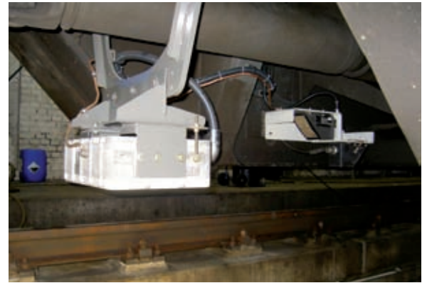
A Euroantenna fixed to the underside of the train for communication with balises.
